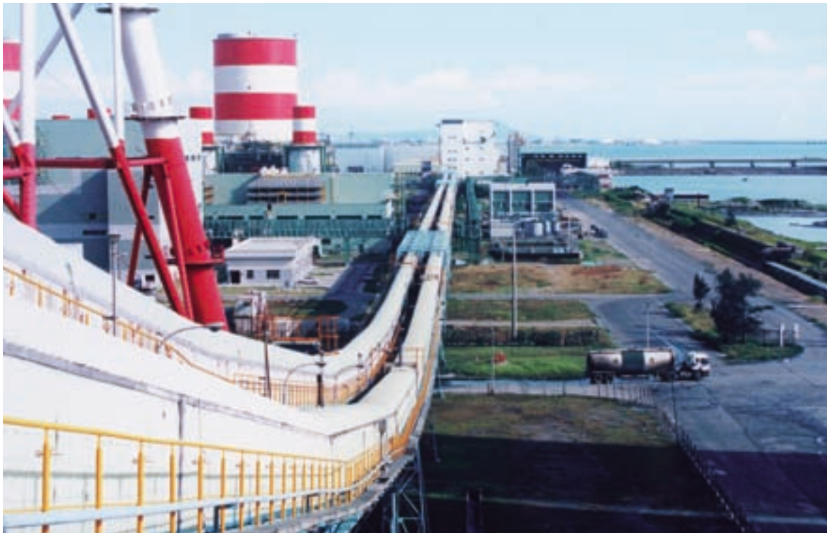
電廠輸送線 Conveyor Line at Power Station
